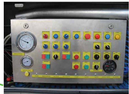
A steel enclosure solution used as a control unit in a sewage truck in Poland.
